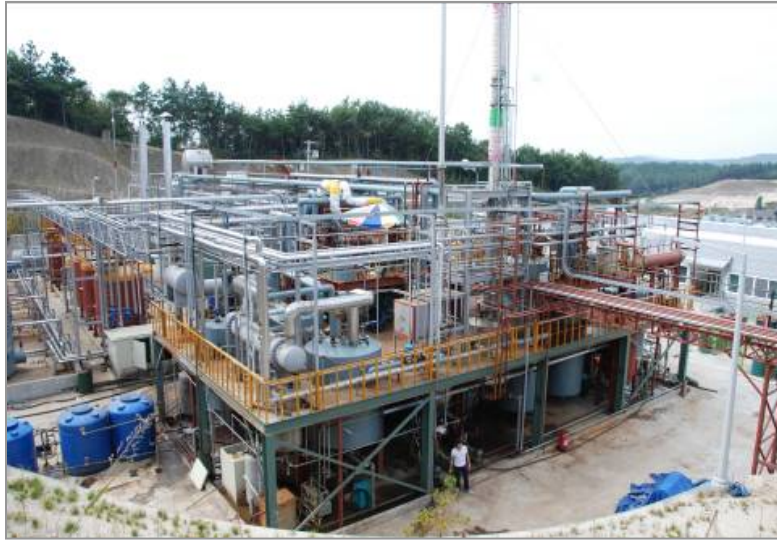
Figure 9. Biodiesel plant employing solid catalyst at Yeosu. Reference: SM-POT
