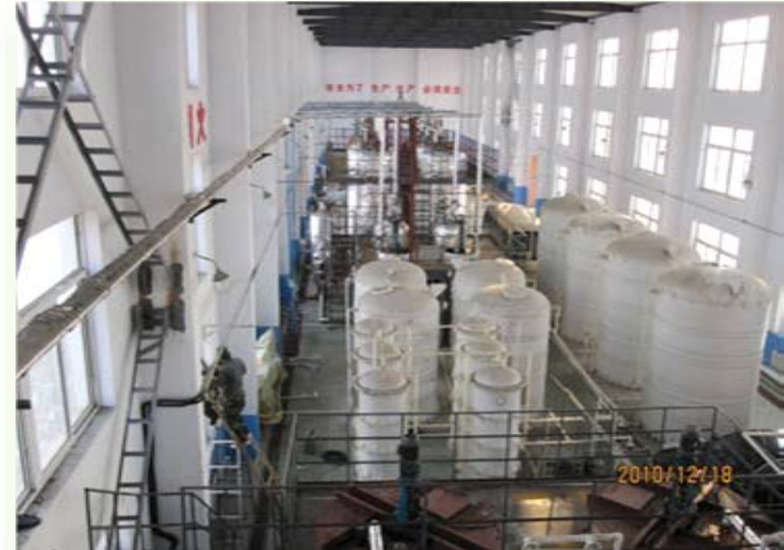
Pilot Plant (Yingkou, Liaoning) Capacity: 165 gallons/day
