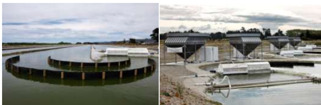
Figure 3. NIWA's 5 ha wastewater treatment HRAP
