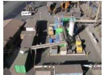
Figure 4. LanzaTech's Glenbrook pilot plant.
